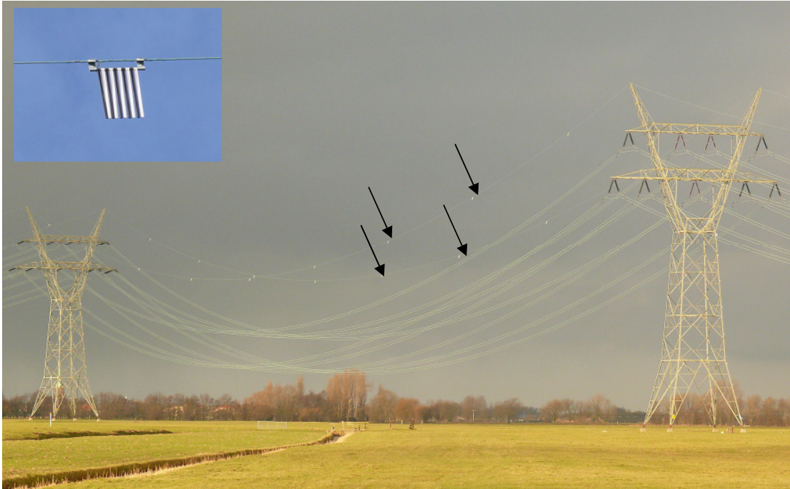
Figure 20. High tension (150 kV) power line in the Netherlands with bird flappers (see arrows) placed at regular intervals in both ground wires as bird flight diverters, see also Box 1 (Photo: Bureau Waardenburg).
