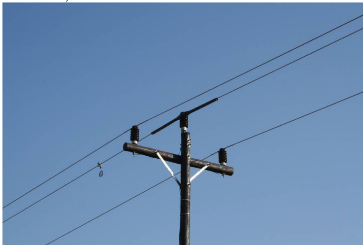
Figure 13. A 'Raptor Protector' used to insulate the centre conductor of a 22 kV pole structure making the distances between non-insulated conductors large enough for safe perching (Photo: EWT-WEP).
