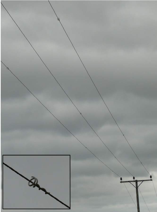
Figure 19. Medium voltage distribution line with small spirals (so-called 'pig tails') placed at regular intervals in the conductors as bird flight diverters (Photo: Bureau Waardenburg).
