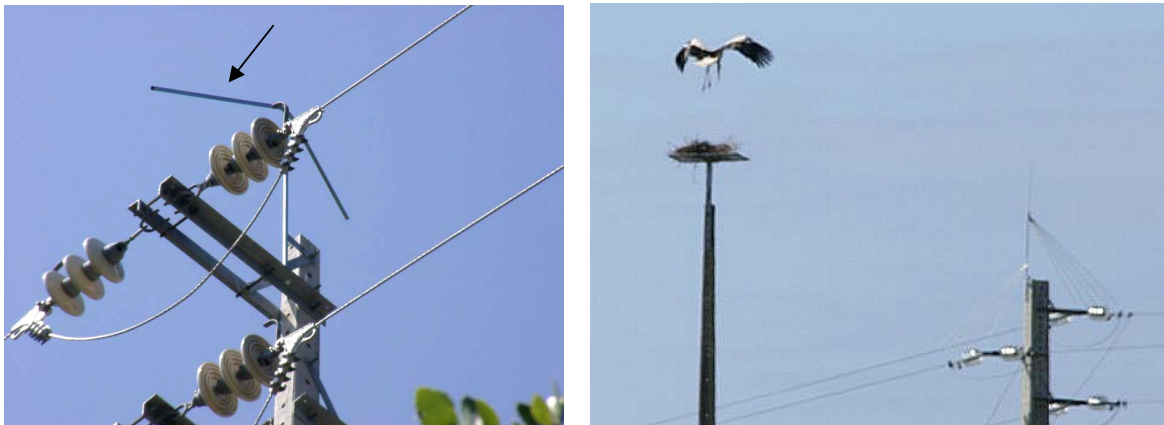
Figure 11. Distribution pole with symmetric chevron (arrow) on top as bird exclusion device (Photo: EDP-Distribution, Portugal; and distribution pole with bird exclusion spikes with dedicated nesting pole for White Stork next to it (Photo: Carlos Tiago).
