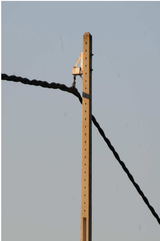
Figure 9. Completely insulated medium tension cable in Spain hanging from concrete pole without need of insulators (source: Haas, 2011).
